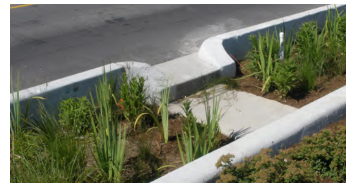
Bioswales treat runoff in Indianapolis
