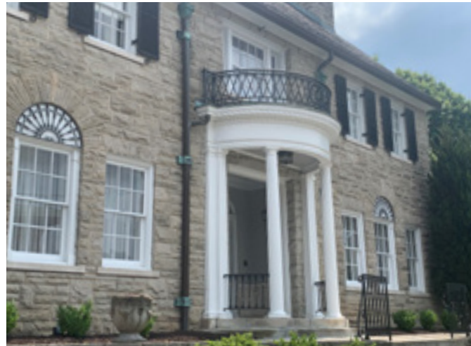
The metal balcony railing and transom grates on the structure above help to define its character and should be preserved.
