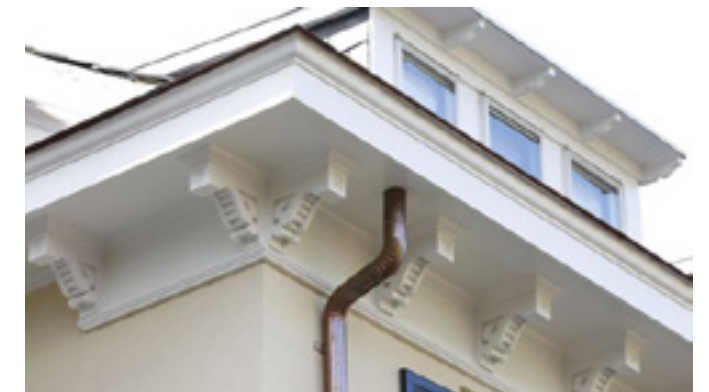
Built-in gutters like those pictured above shall be repaired and maintained.
